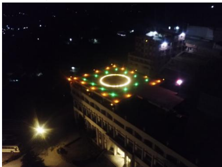
Heliport Lighting on roof of building
